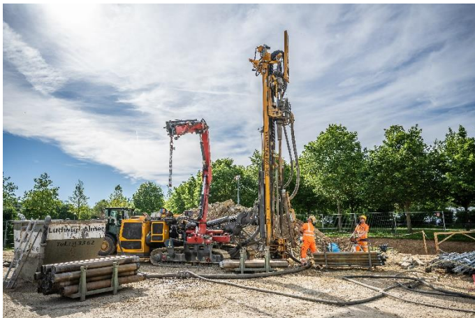
(1) Bauer Resources built a geothermal probe system for the new modular building on the Regensburg University campus in nine months.
