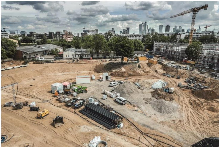
(1) Since January of this year, the Bauer Umwelt Division of BAUER Resources GmbH has been rehabilitating a former industrial site in Frankfurt's Gallusviertel district.
